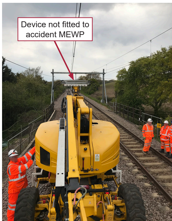
Figure 6: The view from a similar MEWP with the basket slightly raised at the accident location (in daylight)
